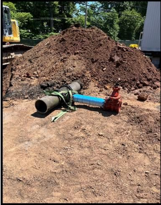
Water Pipe Connection and Valve
