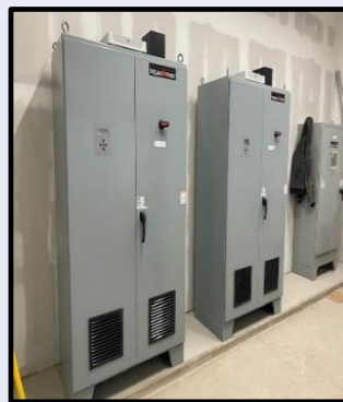
UV/OX Control Panels
