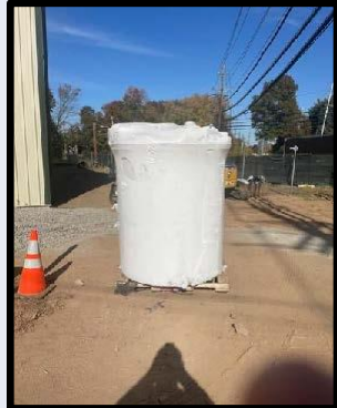
Peroxide Holding Tank
