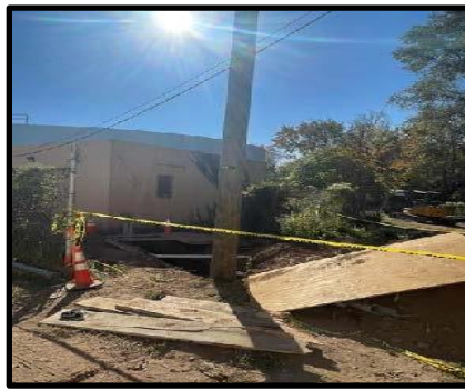
New Power Pole Installed near FL House
