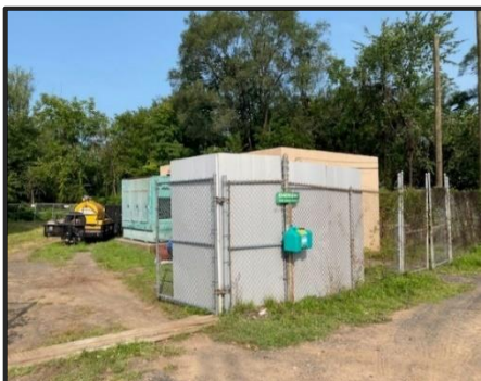
Foam boards to reduce noise from generator
