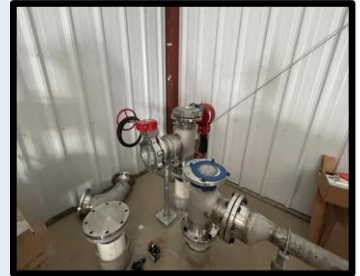
Waterline Piping Connections
