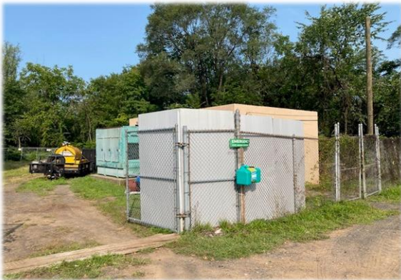
Foam boards around fence to help reduce noise from generator operations
