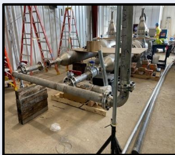
Process Piping to UV/OX
