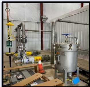
Process Piping to Pumps
