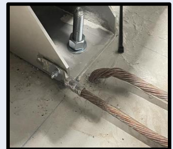
Grounding Wire to Equipment
