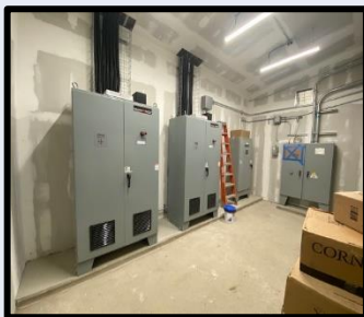
Electrical Room Completed
